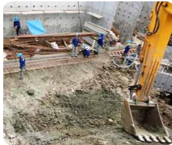
Maynilad is accelerating the construction of its STPs to help protect the environment and the health of its customers.
